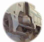
Low & high temp power cables
